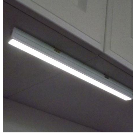
12 inch Daylight White LED Bar 5,000°K
